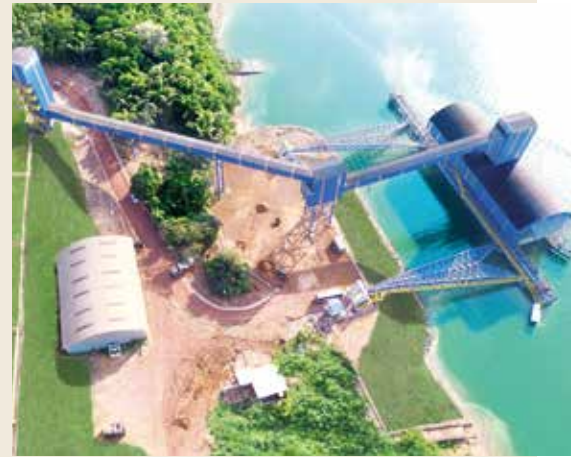
Hidrovias do Brasil S.A project's cargo transshipment station Photography: Rafael Dantas/Hidrovias do Brasil S.A. Collection
